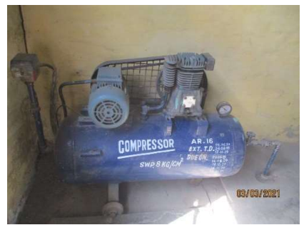
NC Photo # 5 Compressor in unsafe condition
